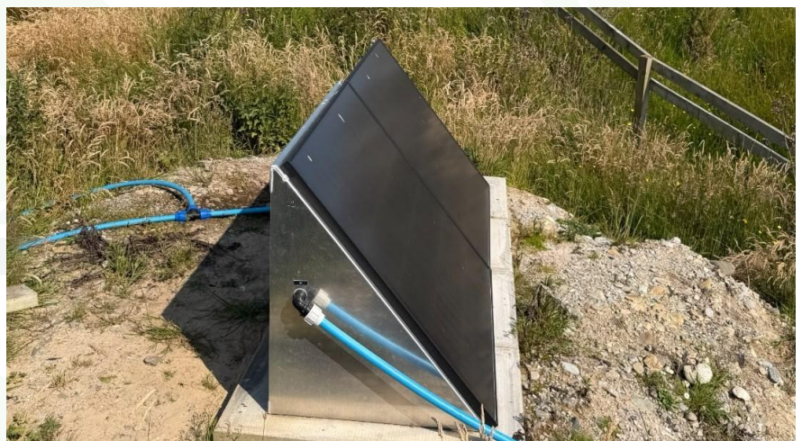
Solar powered water pump from Ardo Water is essential to supply water for the rotational grazing system.
